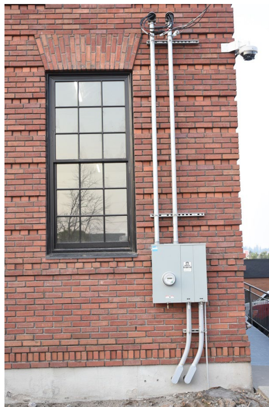
12. New electrical feed on northwest corner
