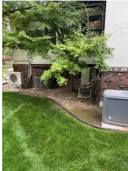
New Generator & HVAC Towers
