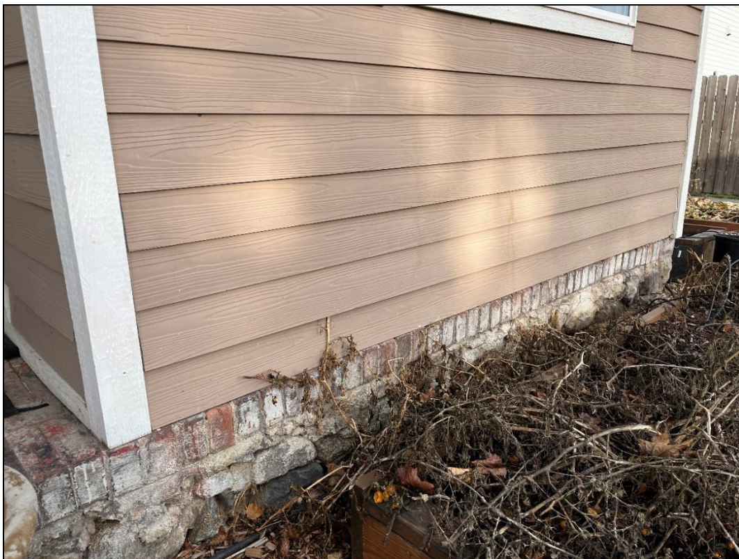
Cook-Abele House rear porch foundation and brick floor where the porch is enclosed on the east end, 12/15/2023. Photo taken by Logan Camporeale SHPO.
