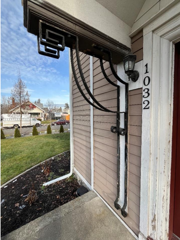
Cook-Abele House wrought iron details on front porch roof, 12/15/2023. Photo taken by Logan Camporeale SHPO.
