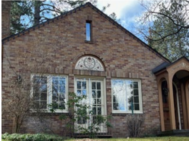
Figure 15: Historic French doors and multi-pane casement windows are fitted with storm sash. W 21st Ave
