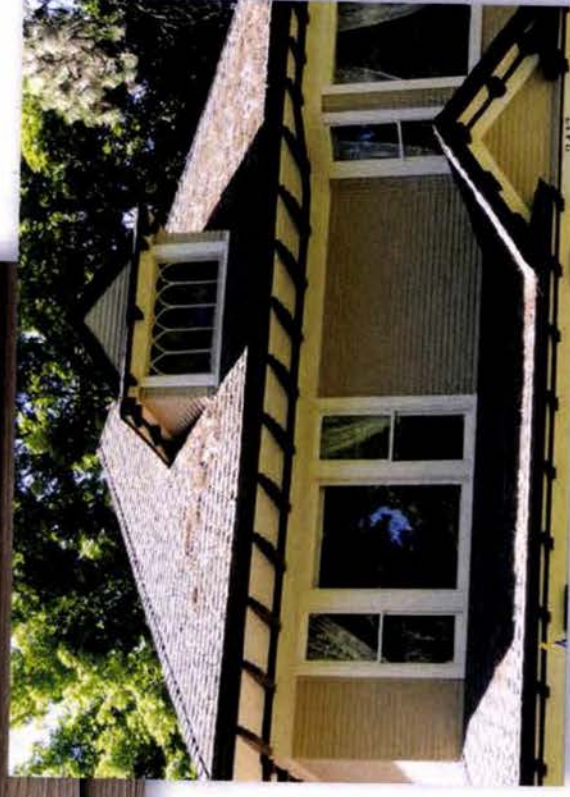
Notice what some composite siding materials look like (above). The false graining is not historically appropriate. The house below has wood clapboard siding which would have originally been sanded smooth and painted, concealing the grain.
