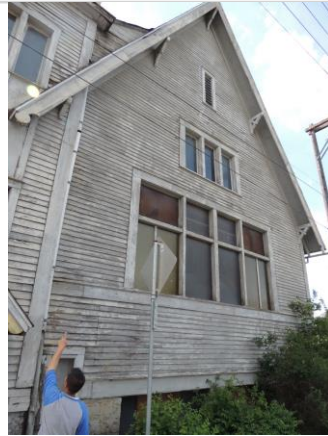
The east facade faces Arthur Street. The main entrance to the church is just to the left, through the 1928 addition. Note decorative bargeboard. Photo taken May 29, 2015.
