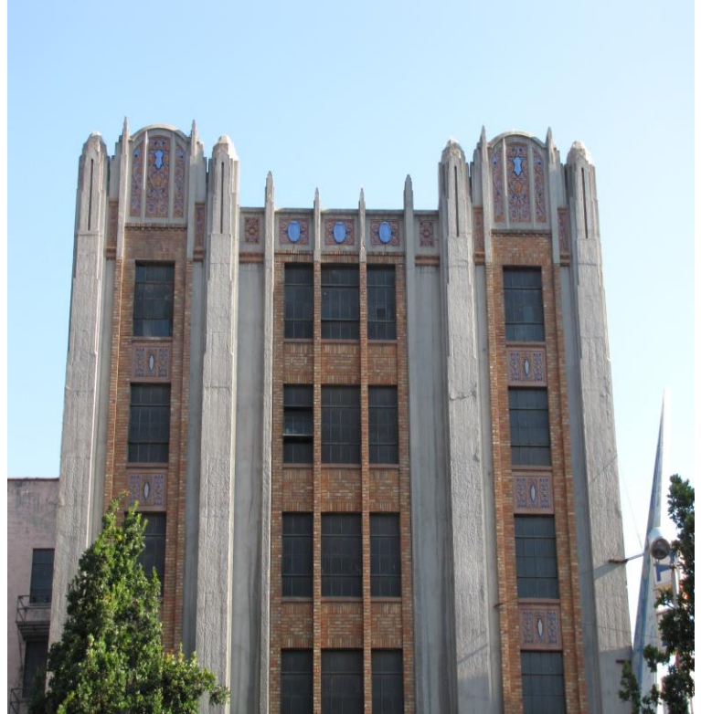
Rehabilitation work continues at the City Ramp Garage at 430 W. 1 st Avenue. The project is being completed with historic preservation incentives.
