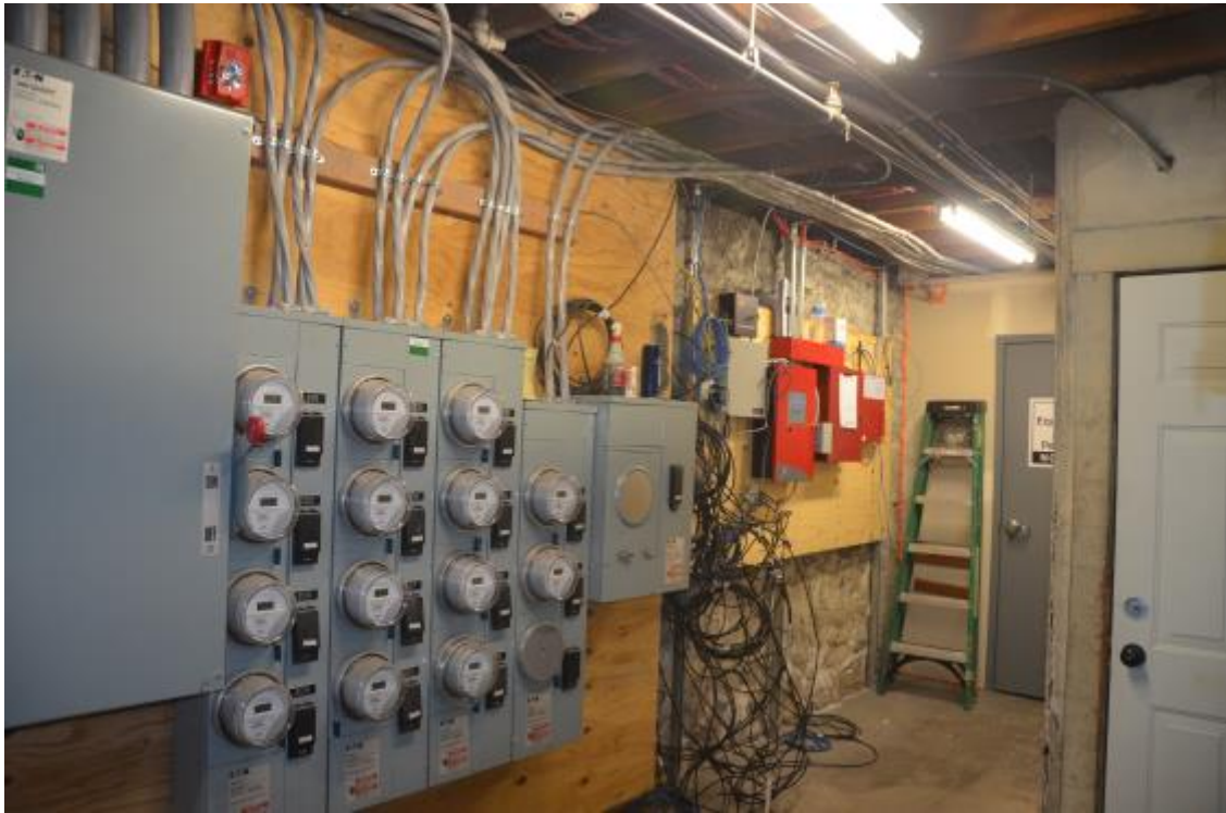
34. Basement - electrical panel – door to upstairs on right
