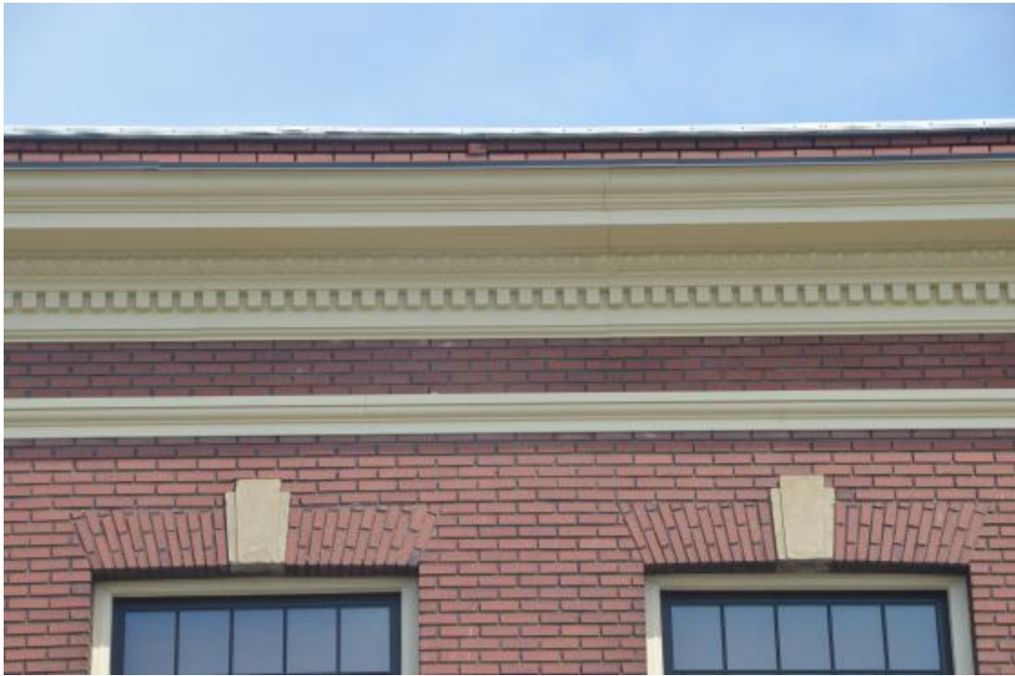
13. Detail of sheetmetal cornice and belt course, and 3rd floor window heads
